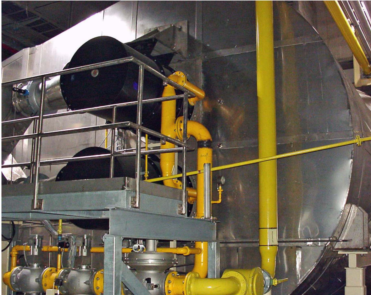
Two gas fired MEGAFIRE® 45M EB burners, total capacity 20 Megawatt heating a recirculating process air stream which feeds a TAD on a paper machine.
